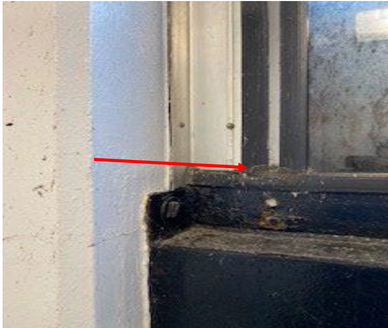
Photograph 3 – A view the asbestos-containing black interior window caulk.
