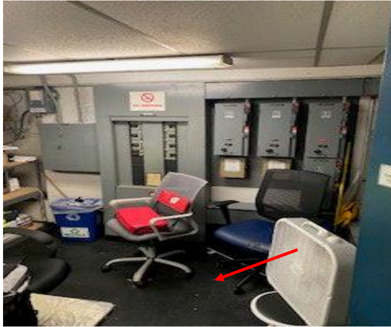
Photograph 1 – A view of the office with asbestos-containing mastic beneath flooring.
