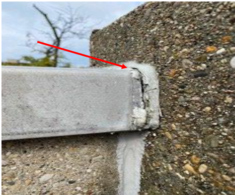
Photograph 2 – A view of the asbestos-containing hard gray parapet caulking.
